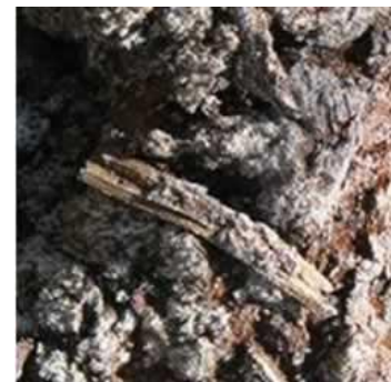
Salt crusts forming on surface
