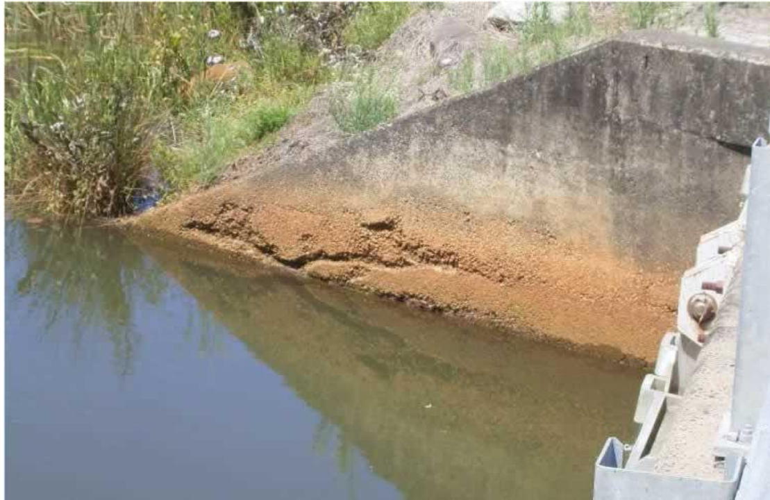
Concrete breakdown and iron corrosion on bridge abutment Murray-Darling Freshwater Research Centre, D. Baldwin
